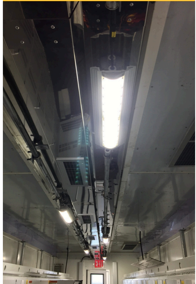
HDL2s in an electrical control room
